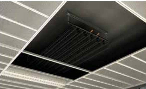
Figure 9: Radiant/convective beam above perforated ceiling
